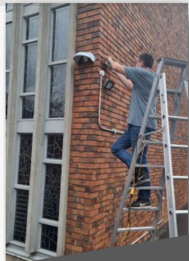
Security camera installed in rear car park
